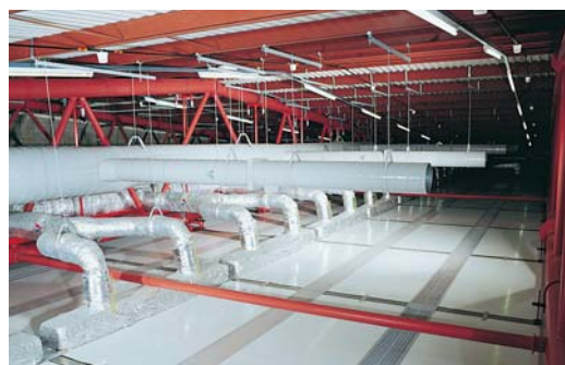
Network Room Roof Void
